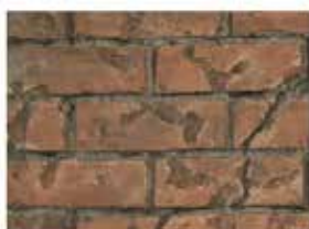
Cracked Red Fire Brick
